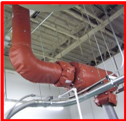
Fabricated cover system for industrial generator exhaust system.
